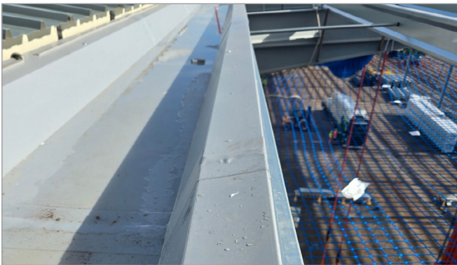
Gutter bearing leg wrapping over purlin at rafter location but not at mid bay as purlin is out of alignment
