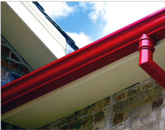
Figure 1: Typical external eaves gutter
