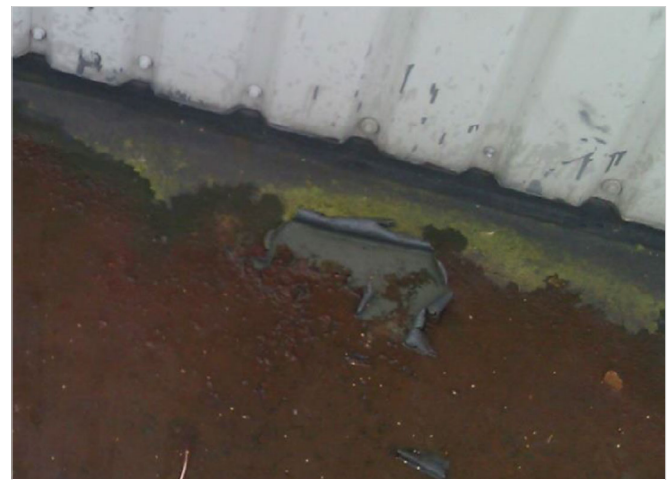
Liquid applied lining material delaminating from the gutter
