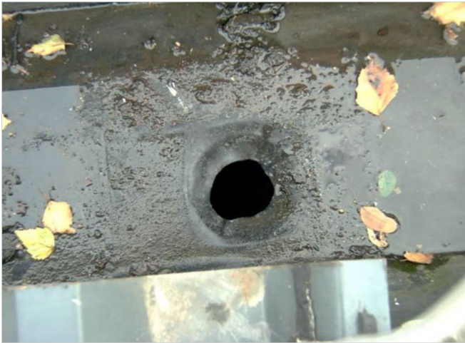
Gravity outlet restricted by installed liners
