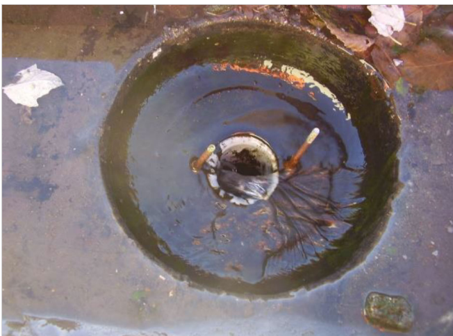
Siphonic outlet restricted by installed liners
