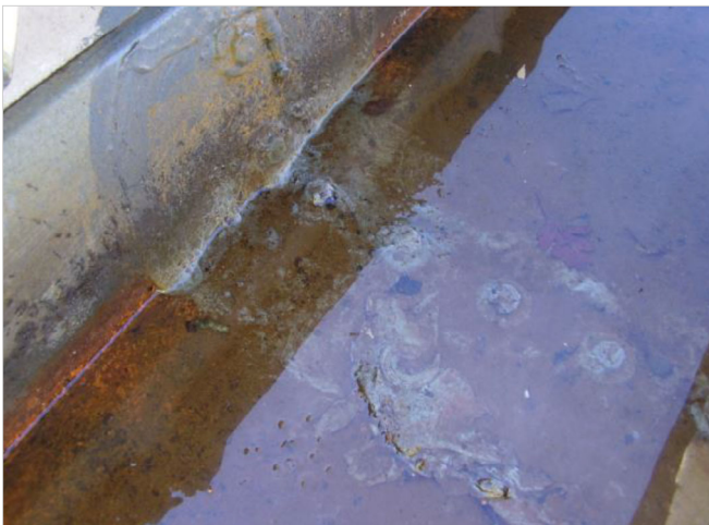
Metal gutter suffering corrosion and joint leakage
