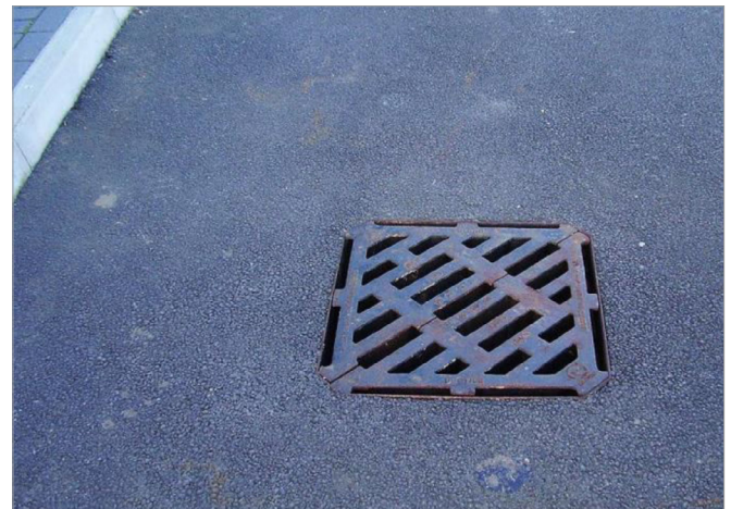
Vented lid on discharge manhole
