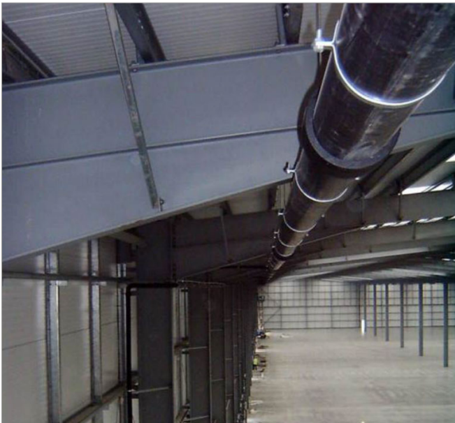
Siphonic pipework horizontal at high level
