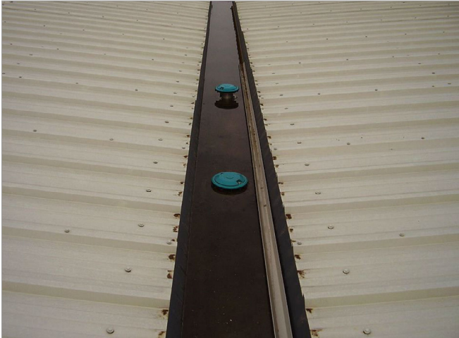
Typical primary and secondary siphonic outlets in gutter
