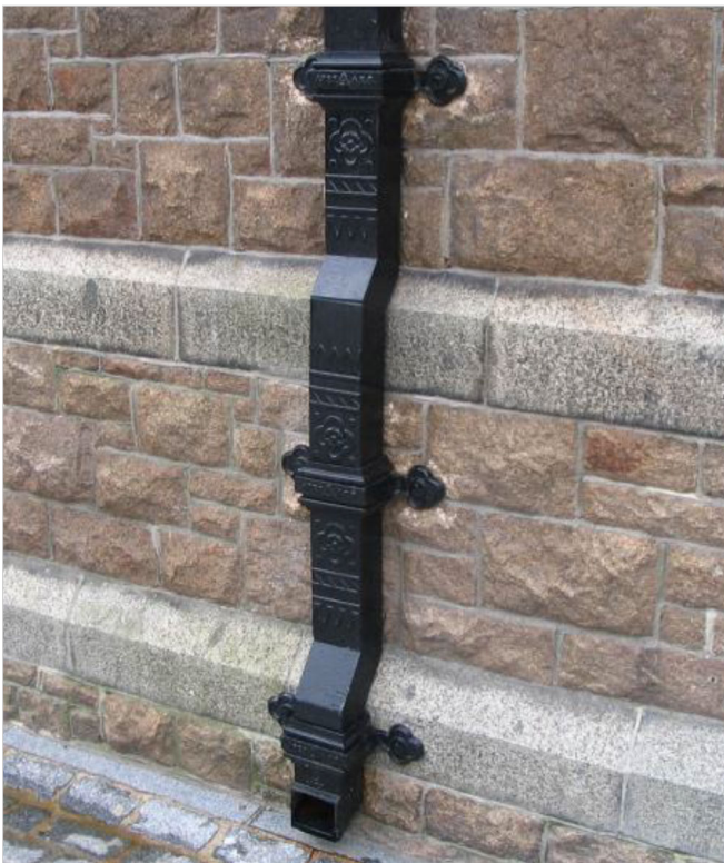
A cast iron drainpipe at Guernsey Market, St Peter Port, Guernsey
