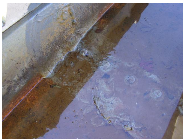
Fig 1 Metal gutter suffering corrosion and joint leakage
