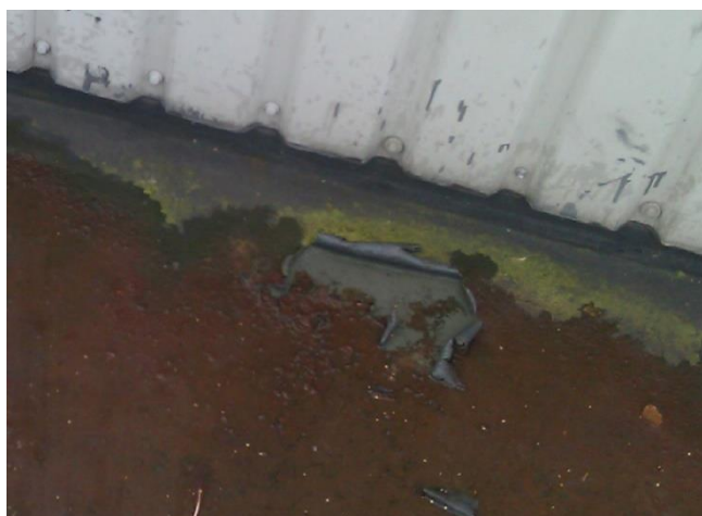
Fig 2 Liquid applied lining material delaminating from the gutter
