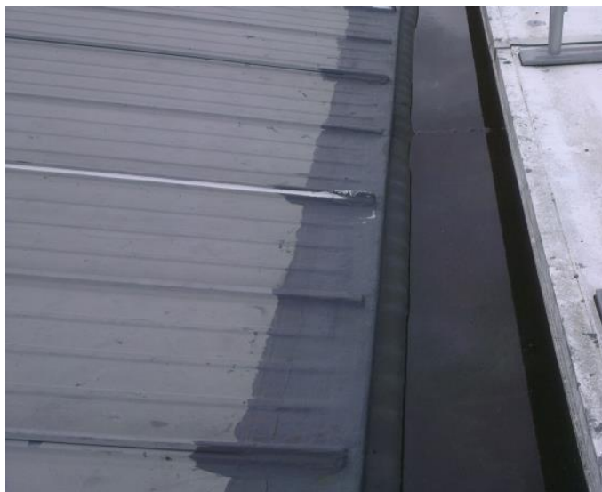
Fig 4 Water trapped below side slope of lining system extended onto roof sheets
