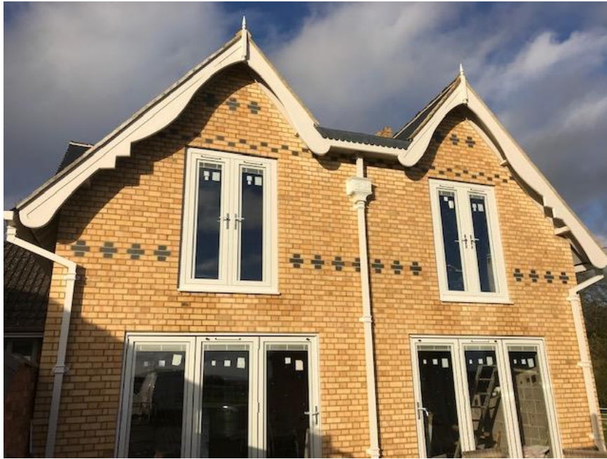
Aluminium hopper and cast square downpipe
