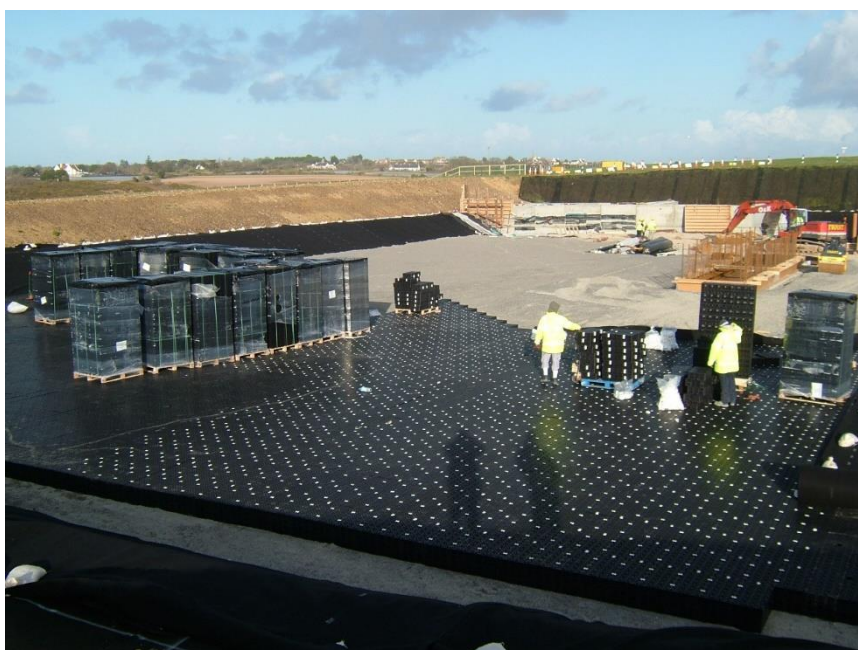
Many sites now have underground storage tanks which, if poorly detailed, can restrict discharge from roof drainage systems
