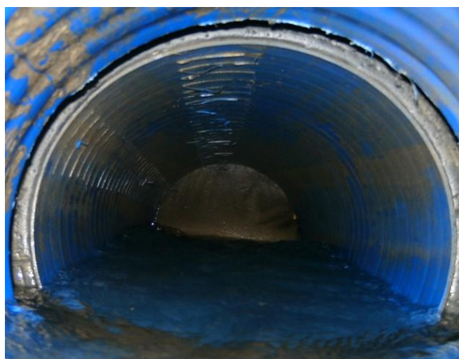
Poor detailing in SuDS tank (geotextile not trimmed away at pipe entry) limiting flow
