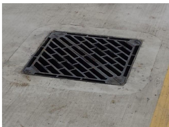
Vented manhole lid for siphonic system
