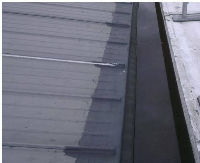
Fig 4 Water trapped below side slope of lining system extended onto roof sheets
