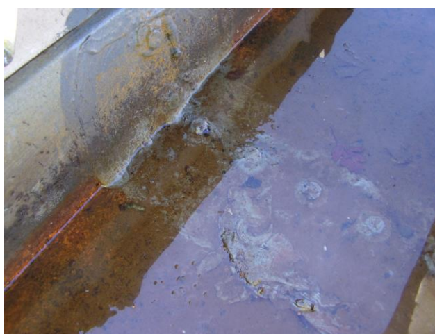
Fig 1 Metal gutter suffering corrosion and joint leakage
