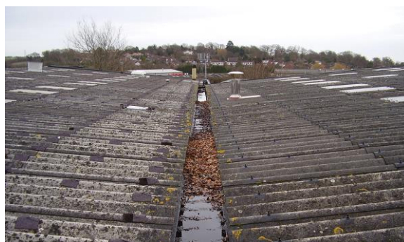
Even good designs will fail if not maintained
