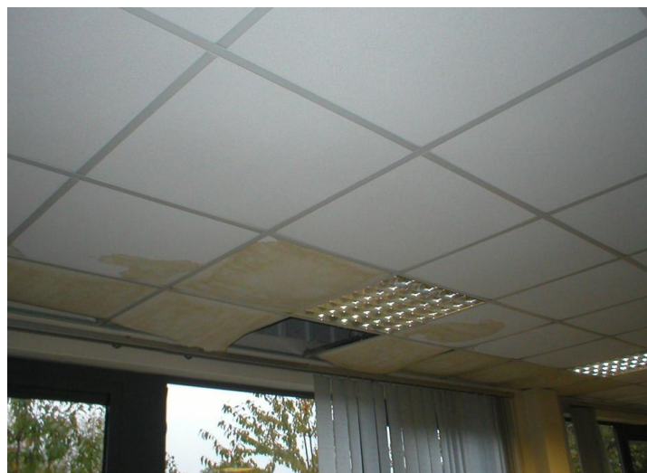
Damage caused by inadequate roof drainage
