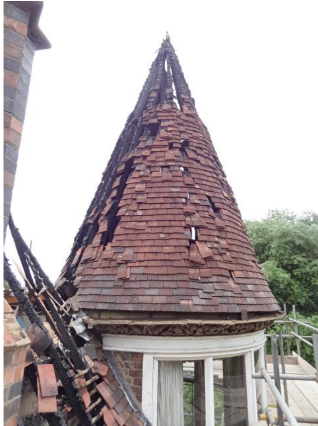
The turret in need of repair
