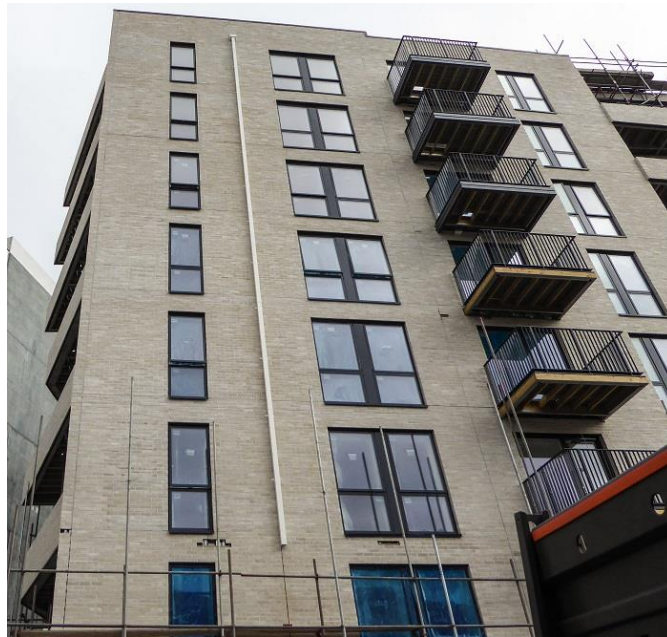
Neat collars of rear fixing pipe clips provide clean lines
