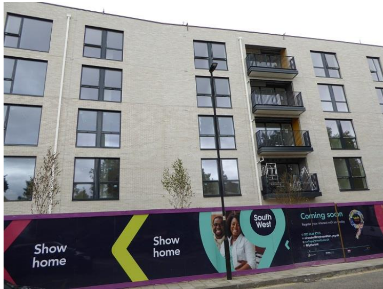
Guttercrest rainwater hoppers and downpipe at SW9
