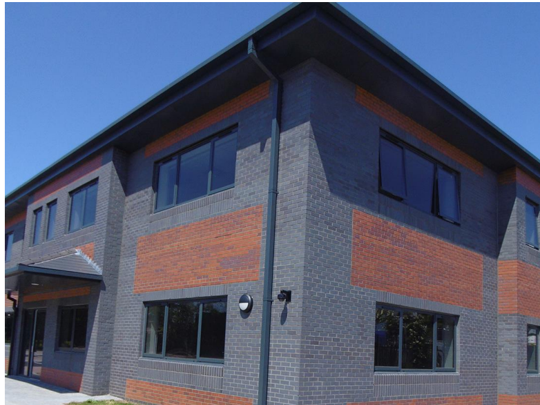
Aluminium box gutter and rainwater pipes Image courtesy of ARP Limited
