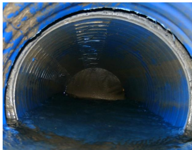
Poor detailing in SuDS tank (geotextile not trimmed away at pipe entry) limiting flow
