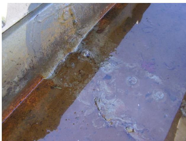
Fig 1 Metal gutter suffering corrosion and joint leakage
