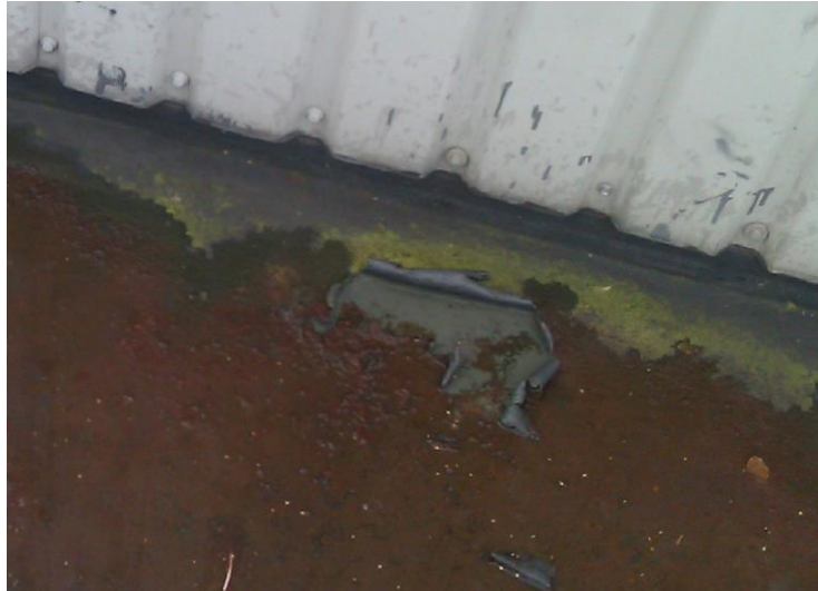
Liquid applied lining material delaminating from gutter
