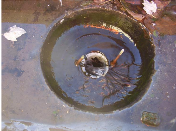
Lining fitted to siphonic outlet restricting performance
