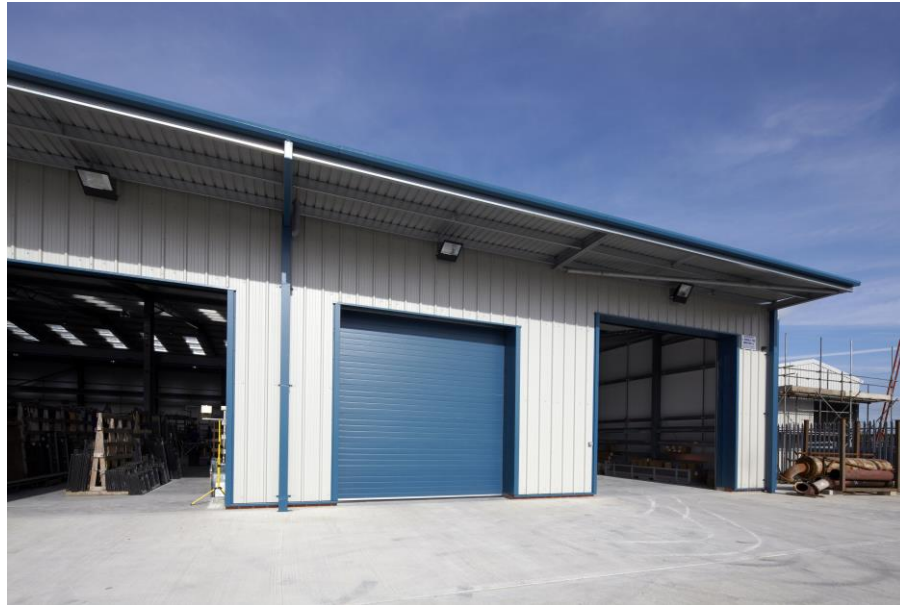
Steel guttering installed at Northern Glass Express, Fleetwood. Courtesy of A Steadman & Son
