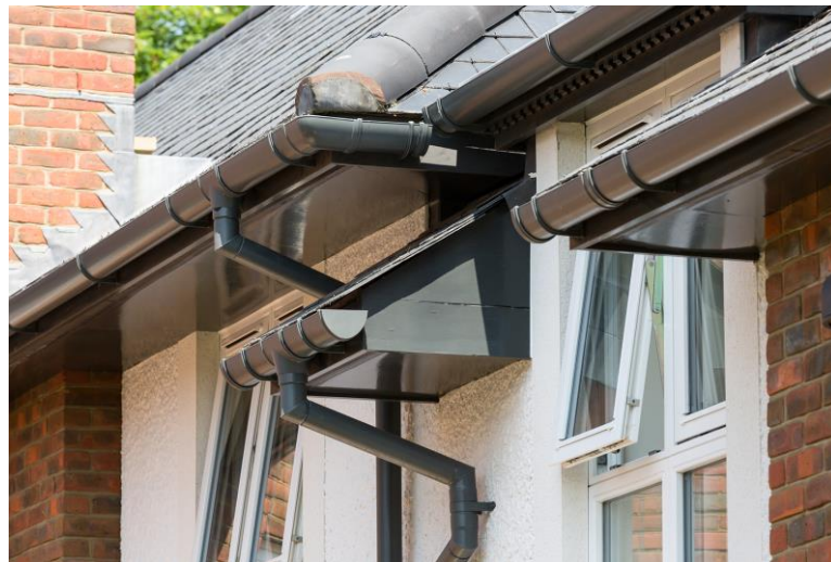
Aluminium rainwater system installed at St Catherine's Dementia Care Home, Winchester Courtesy of Alutec
