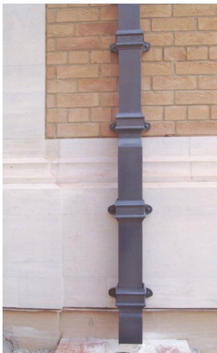
Cast iron downpipe. Centre for Islamic Studies, University of Oxford Courtesy of Hargreaves Drainage
