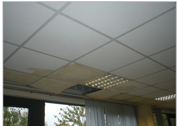
Damage caused by inadequate roof drainage
